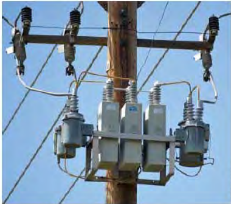
Figure 5.34 Three-phase capacitor bank.
