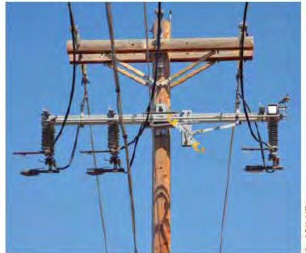
Figure 5.24 Open airbrake switches.
