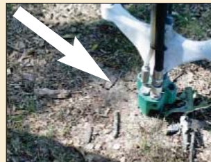
Figure 17. Reducing soil compaction using high-pressure air injector. Cracking of soil indicates some relief from compaction.
